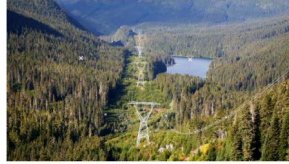
North Coast Transmission Line, Northwest British Columbia
