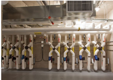
2,800 various other assets (electrical, mechanical, water and drainage systems)
