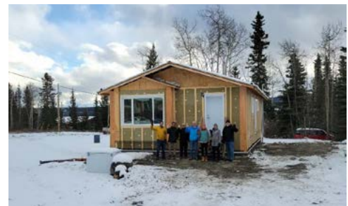
NRC researchers, the Arctic and Northern Challenge program team and representatives from Earthrise Building Services and Champagne and Aishihik First Nations toured retrofit projects underway.
