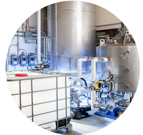
Anaerobic Bioprocesses Pilot Plant at Royalmount
