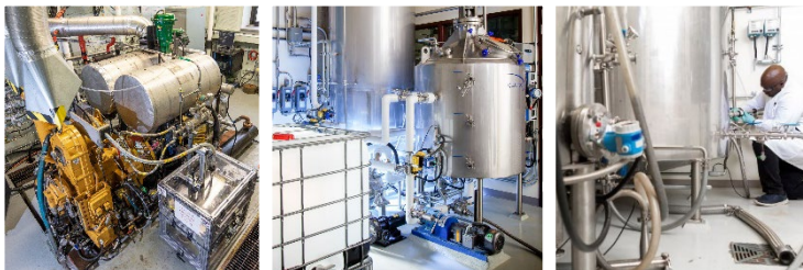
Ottawa's hydrothermal conversion equipment and Royalmount's biomining and bioprocess facilities equipment
