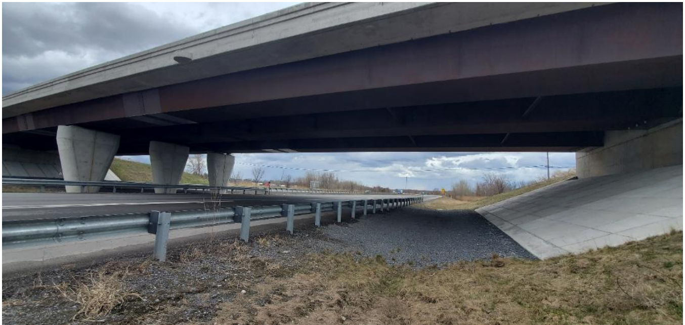
Figure 5-13. Field perspective of the Highway 401 Underpass at County Road 2 & County Road 34 I/C. The image illustrates the primary installation environment, featuring weathering steel girders and reinforced concrete piers. Sensor plates are strategically distributed across these structural elements, including the abutment (right), the central piers, and the girder webs over the traffic lanes, to capture varying degrees of exposure to roadway splash and aerosolized de-icing salts.
