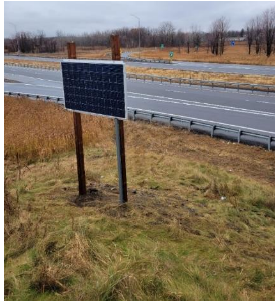
Figure 5-20. View of the autonomous solar power system. The panel is mounted on a rigid support structure on the south-facing embankment to provide a continuous renewable energy source for the bridge's remote monitoring and data transmission instrumentation.
