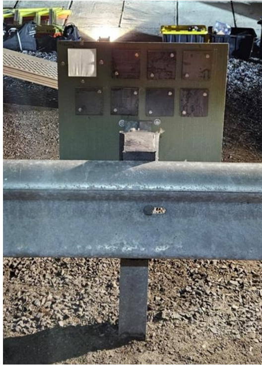
Figure 5-22. Close-up view of the mounting plate secured to the rail post. This station holds a series of weathering steel (WS) mass-loss coupons, specifically configured to monitor the corrosive impact of seasonal variations and roadway splash at the structure's exterior boundary.
