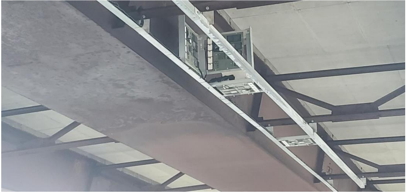
Figure 5-24. Detailed view of the monitoring stations installed on the primary mounting rail over the acceleration lane and #2 middle lane. In the foreground, the Plate 3 cluster evaluates the influence of orientation on corrosion rates above the #2 middle lane: Plate 3.1 faces downwards, Plate 3.2 is mounted vertically and parallel to traffic, and Plate 3.3 is mounted vertically and perpendicular to traffic, directly facing oncoming flow. In the background, at the farthest extent of the rail, Plate 2 is positioned to monitor the micro-climate specifically associated with the acceleration lane.
