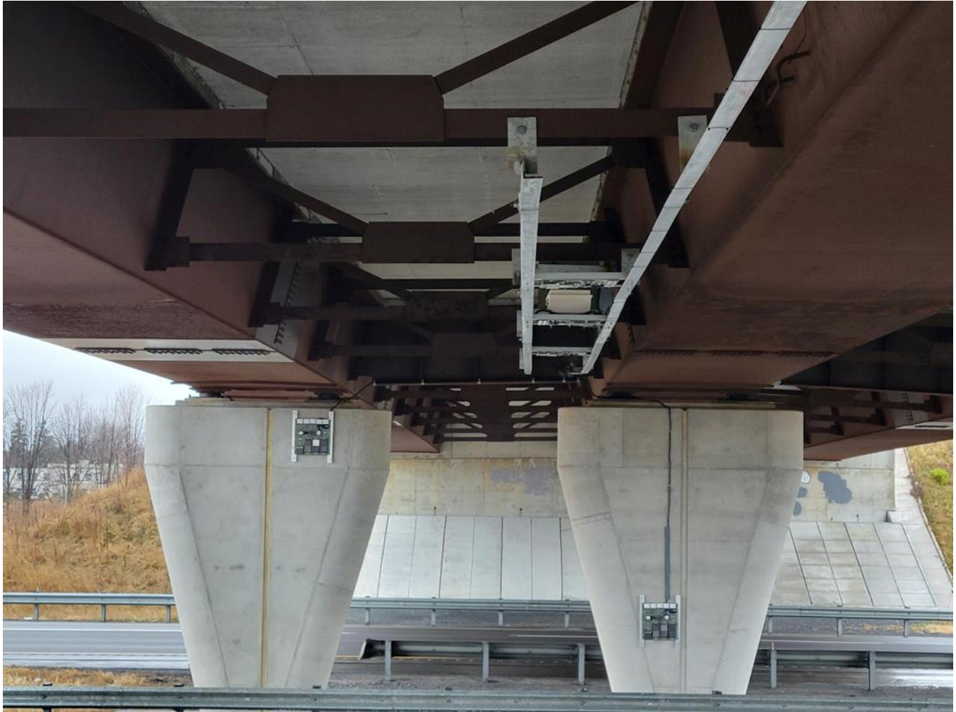
Figure 5-26. Interior view of the bridge superstructure highlighting the instrumentation mounted on the reinforced concrete support piers. Plate 5 is installed on the lower section of the second pier (right), positioned at a standardized "splashing height" to monitor high-intensity roadway runoff. Plate 6 is secured to the upper section of the first pier (left), near the girder interface, to evaluate the corrosivity of the environment at a higher elevation. The central mounting rail and its associated over-lane sensor clusters are also visible, illustrating the vertical and horizontal distribution of the monitoring network.
