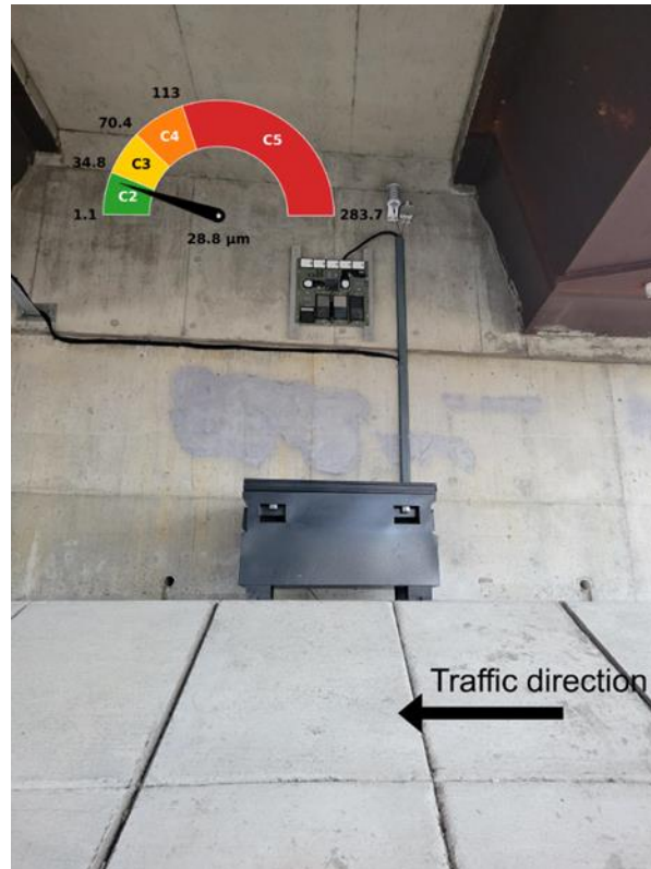
Figure 5-55. In-situ monitoring results for the weathering steel sensor installed on the Right abutment wall (panel 1).
