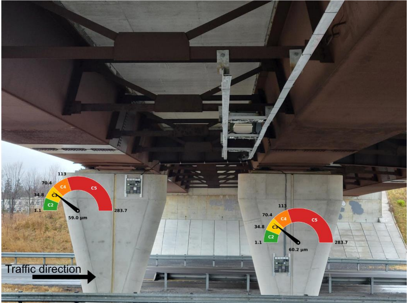
Figure 5-57. In-situ monitoring results for the weathering steel sensors installed on the bridge piers (panels 5 and 6).
