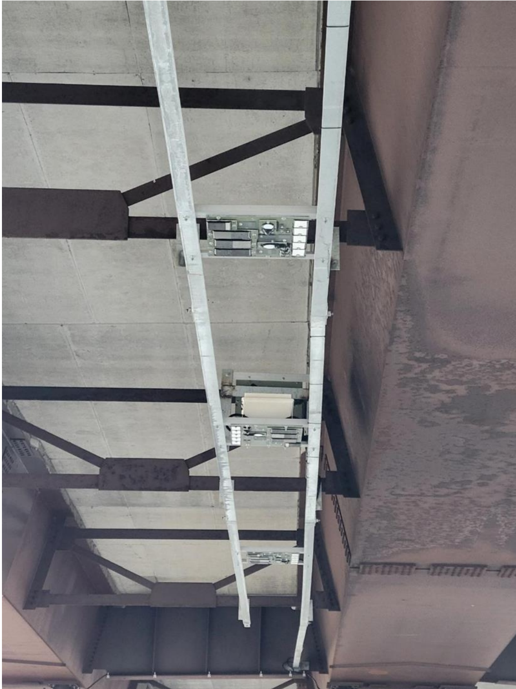
Figure 5-25. Interior longitudinal view of the mounting rail system spanning the primary bridge girders. The image illustrates the sequential positioning of the instrumentation stations from front to back (top to bottom of photograph): Plate 2 (situated above the acceleration lane), the Plate 3 cluster (above the #2 middle lane), and Plate 4 (at the farthest extent above the #1 left lane). This alignment ensures that the monitoring network covers the full width of the traffic-induced spray.
