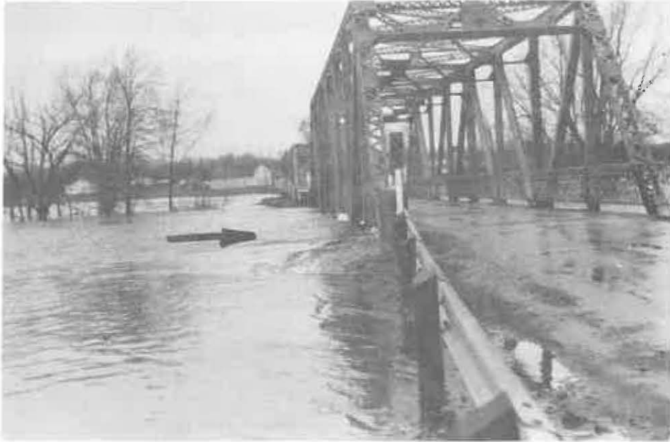
Lakeville Corner Bridges, water level is almost at bridge deck, May 1, 1979, at 10:40 a.m.
