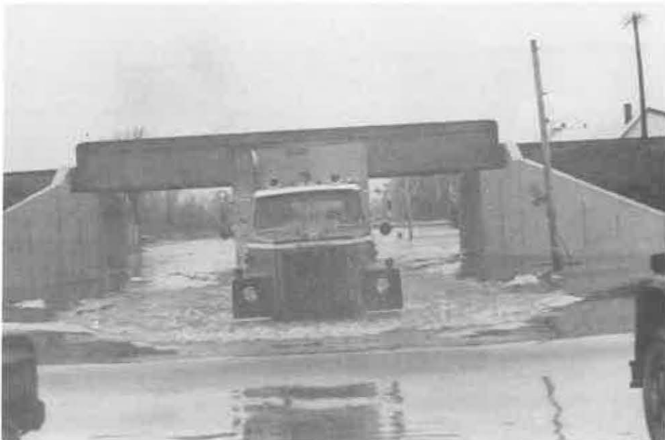
Devon Underpass on the north side of the Saint John River at Fredericton, May 1, 1979, at 1:00 p.m.
