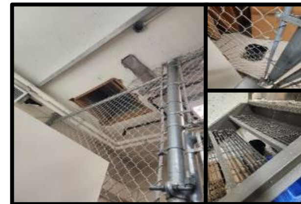
Images of water intrusion in the Edmonton lab's evidence recovery storage
