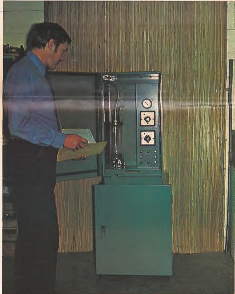
Sirco Controls' B/ST-VS Series raw sewage sampler is shown just before start-up in a municipal sewage treatment plant.
