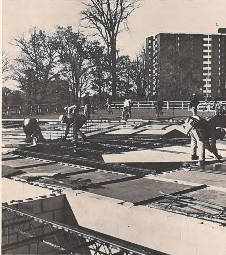
Workmen using the Hambro D-500 Composite Floor System at the site of an apartment development.
