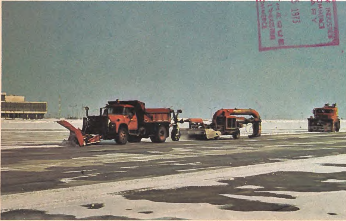
The airport team—plow with sweeper attached followed by a snow blower. Airport runways must be cleared to the blacktop and the sweeper removes the thin layer left by the plow. The steel bristled tubular sweeper has its own power unit with a fan and adjustable air ducts that can be used to blow away the light drifts of snow left by the sweepers action, and to clear the runway lights. Code I-1
