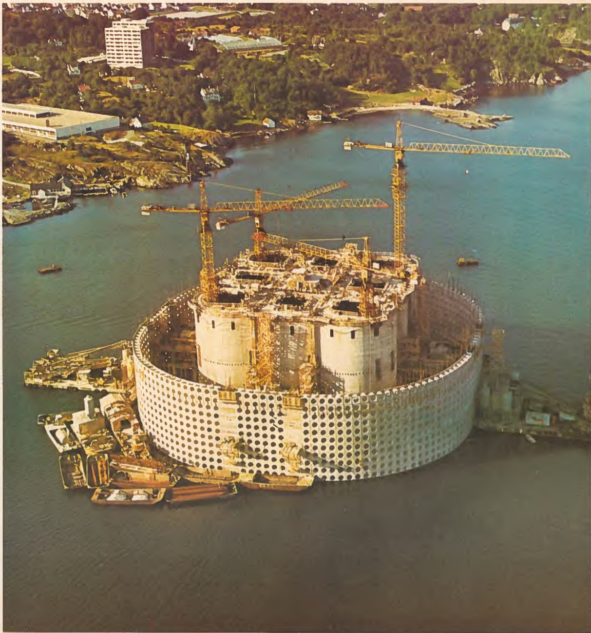
Based on a Canadian invention, this artificial oil storage island under construction in Norway is to be installed in the North Sea. The storage tank, which provides stable deck areas, will sort crude oil at the offshore drilling site. The sea platform design could also be used to provide marine bases for oceanographic studies or as offshore nuclear power plants.
