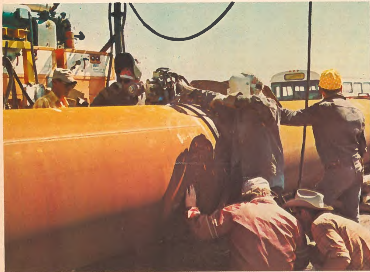
Employees of Alberta Gas Trunk Line Company are shown automatically welding 42-inch (106-cm) pipe.
