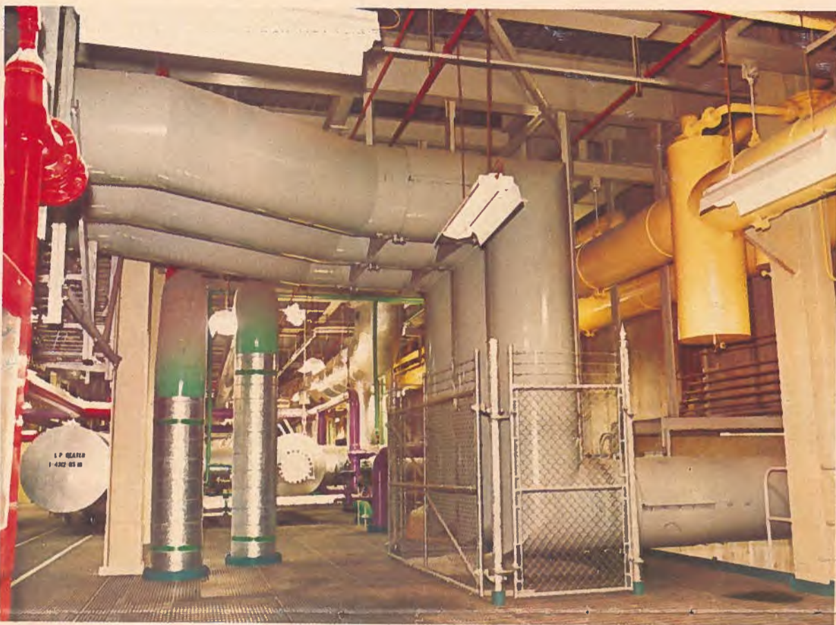
Carrying electric power from the generator to the transformers is this forced-cooled I-T-E Isolated Phase Bus at Ontario Hydro's Pickering Nuclear Generating Station. The Isolated Phase Bus, used throughout the world, is engineered and manufactured by I-T-E Circuit Breaker (Canada) Limited, Mississauga, Ontario.
