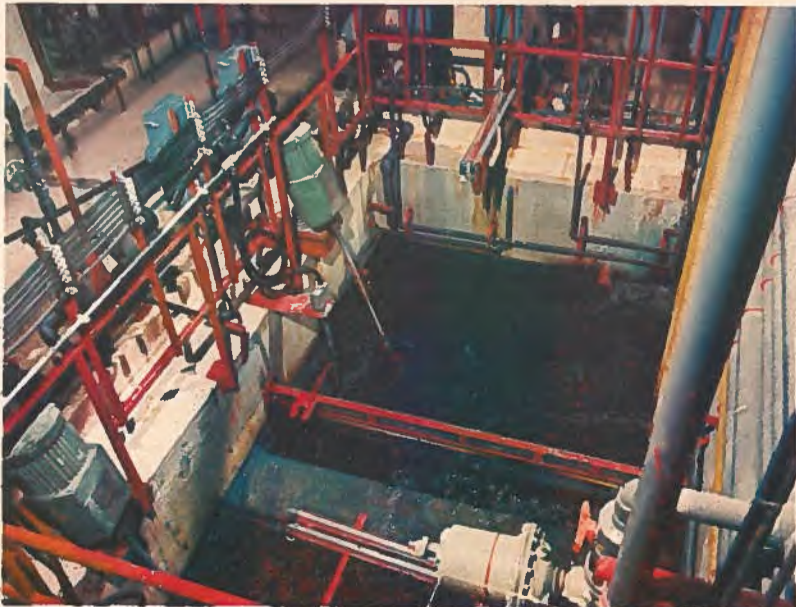
After effluents have been treated for toxicity on Air Canada's aero-engine maintenance base, they are brought together in this neutralization pit. Here the pH is adjusted and all heavy metal hydroxides are precipitated in the form of sludge. The waste treatment system was designed by Surveyor, Nenniger & Chênevert Inc.
