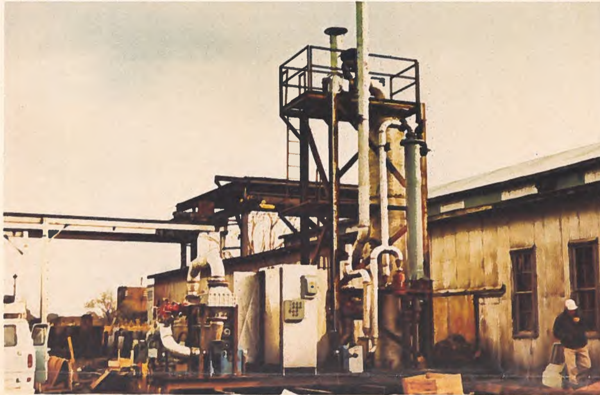
An incineration system for pulp mill odor control installed by Chemetics International Limited.
