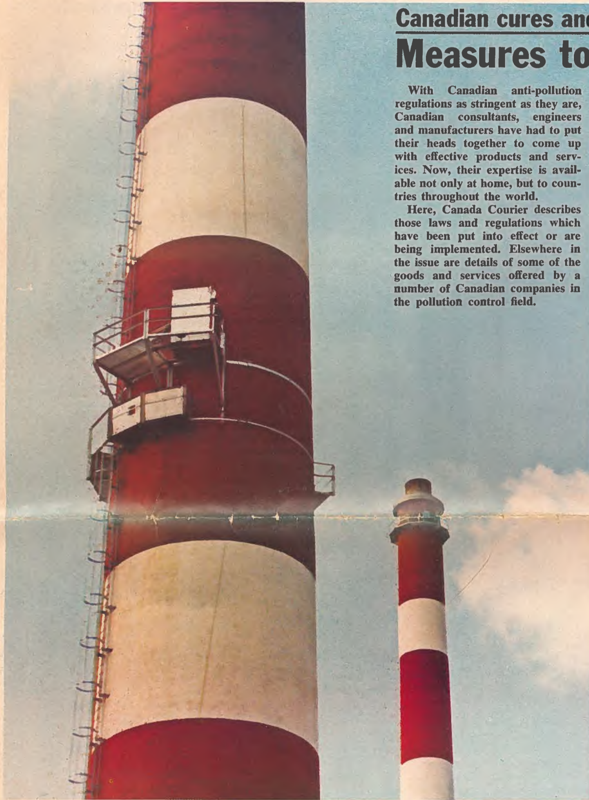
This Canadian system gives a continuous mass emission monitoring of pollutants from an industrial stack. See Western Research & Development story on page 4.
