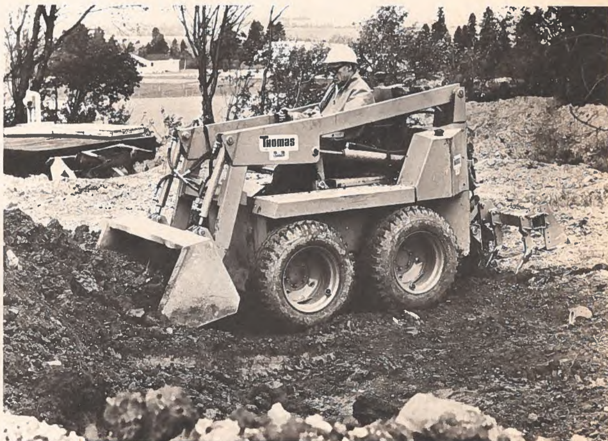
Thomas Equipment's new S/S 700 loader digs dirt with a general bucket on a residential housing construction site at Florenceville, New Brunswick. Scarifier, used for breaking up earth's surface, is attached to rear of unit. This compact, versatile and speedy machine has more than 30 choices in buckets and attachments.
