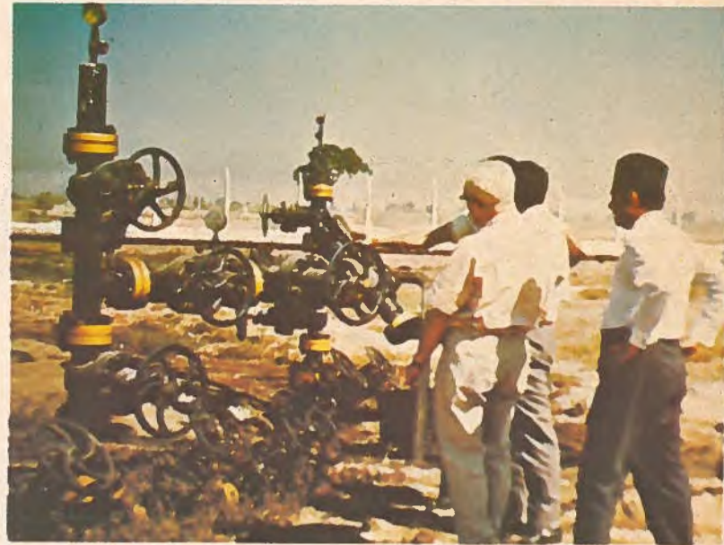
Canadian consultants have extensive experience in the management and direct supervision of drilling operations in such diverse categories as remote Arctic wildcats, offshore wells, deep wells in the highly faulted foothills of Western Canada and wells drilled for thermal recovery operations. This producing wellhead assembly is in India.
