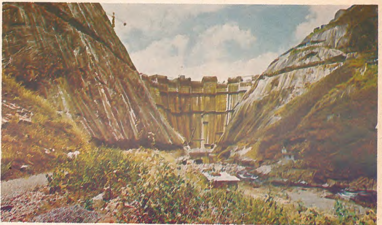
Canadian engineering consultants excel in the power sector. Here construction is being done on the 555-foot (169-m) high Idikki Dam in Southern India. The largest of three dams in a hydroelectric project that will produce 780,000 kilowatts of power at full capacity, the Idikki Dam is a thin, double curvature parabolic concrete arch tapering from a thickness of 25 feet (7.6m) at its crest to 75 feet (22.8m) at its base. It is 1,250 feet (381m) long.
