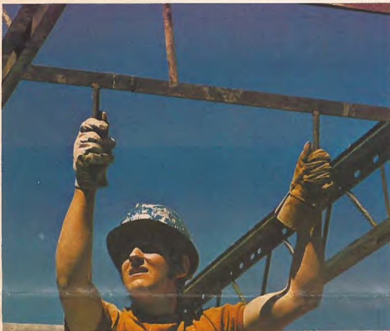
A workman using Hambro's D-500 composite structural floor system places a re-usable roll bar into the slots in the upper member of the joist. Once the concrete deck is set, these bars are rotated for removal of the forms. The floor system, popular in many countries, has also been used with masonry walls, poured concrete walls and in steel framed construction. Code 3-6
