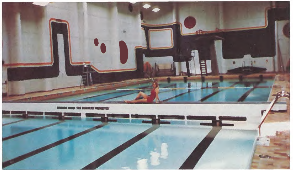
Versatile and economical best describe swimming pools equipped with moveable bulkheads from Dominion Aluminum Fabricating. By relocating the bulkhead, a 51-metre pool can be transformed into a 15-metre pool so athletes can train in the exact conditions they will find in competition pools.
