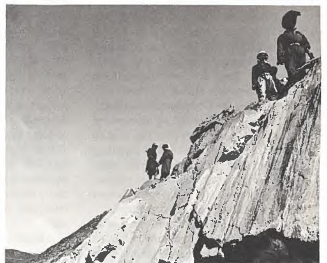
Here workers are seen drilling holes for explosives to widen the trail on the flanks of the Tazadit ore deposits in Mauritania. Development of the deposits was made possible by a World Bank loan.
