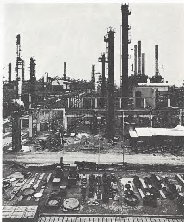
This is the new Petroquimica Uniao complex at Capuava in the state of Sao Paulo where production will begin this year of basic petrochemicals from naphtha.
