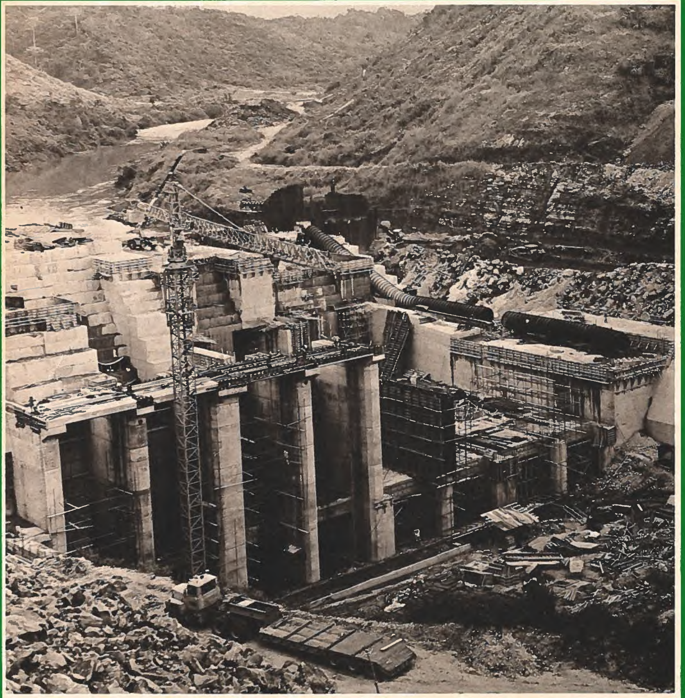
The partly constructed Bayano hydroelectric dam in Panama. Both design and supervision of the work is in Canadian hands.
