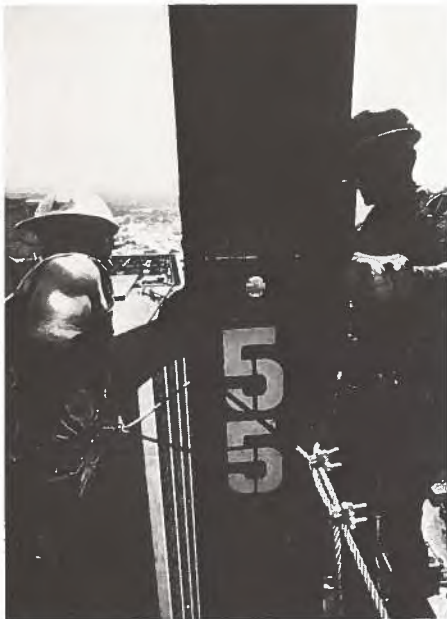
Construction workers guide another girder into place high above the surrounding urban scene of Dallas to keep pace with the most vibrant growing economy in the U.S. — that of the southwestern sunbelt.
