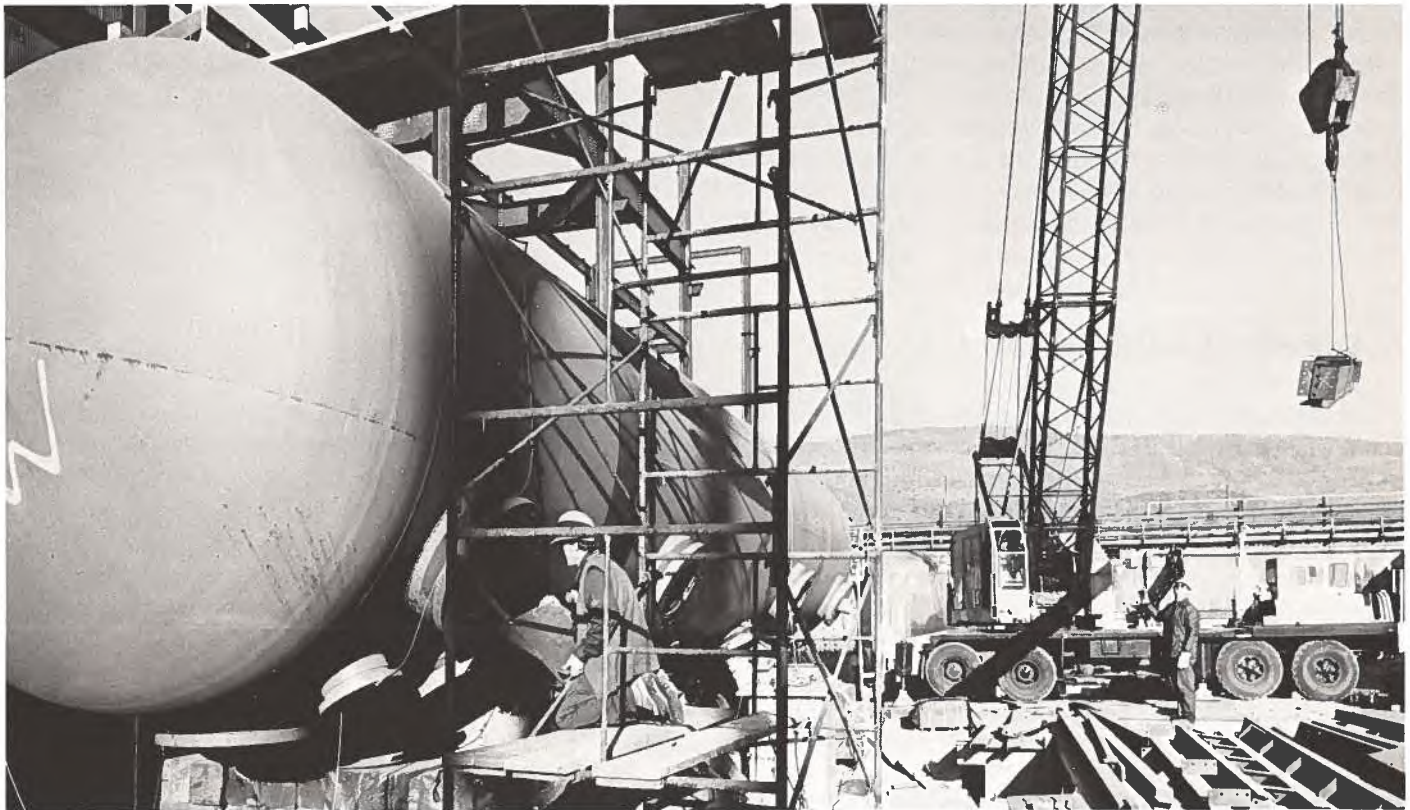
Workman ease the autoclave into its cradle in preparation for righting it into its final resting place as the central piece of equipment in the Sherritt-Gordon-Cominco process for pressure leaching of zinc.
