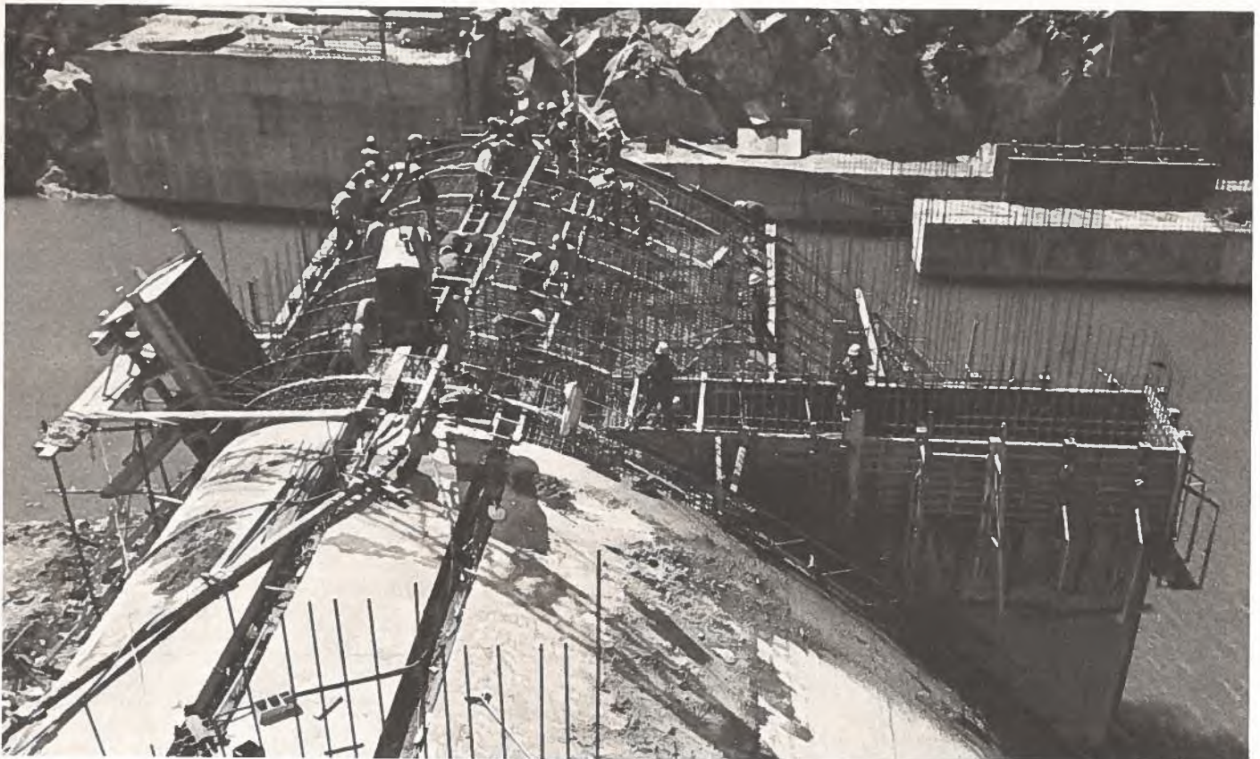
The Foundation Company of Canada is one member of the international consortia involved in the massive Majes hydroelectric-irrigation project in Peru.
