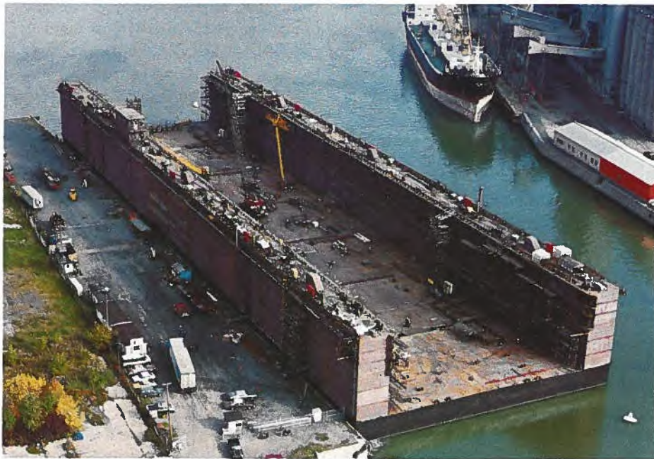
Assembly of the huge PANAMAX drydock nears completion at the Marine Industries Ltd. yards, Tracey, Sorel, Québec. The drydock, 257 metres (843 ft.) long by 52 metres (170 ft.) wide and 20 metres (65 ft.) high, was recently towed down to Halifax where it is being installed as a permanent fixture.
