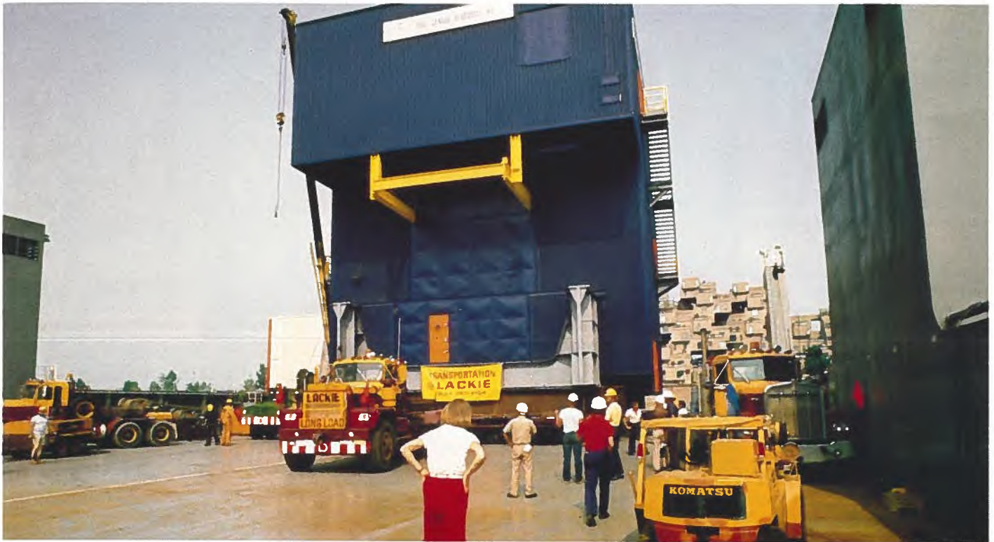
The drilling module, weighing almost 750 tons is eased onto the vessel, Sea Bridge , which will carry it from Montreal to Japan where it and its companion modules will be assembled on the massive steel caisson being built in Japan. The module houses the equipment and services directly related to the drilling activities and is designed to accommodate minor movement by a hydraulic jacking system.
