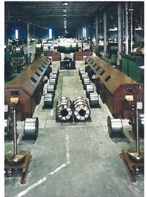
Tubular strander lines designed to accommodate 26" bobbins
