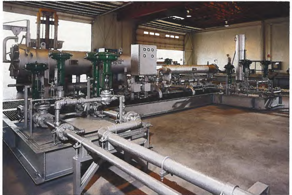
New Zealand-bound gas compressor station can be operated and monitored remotely by telemetry.
