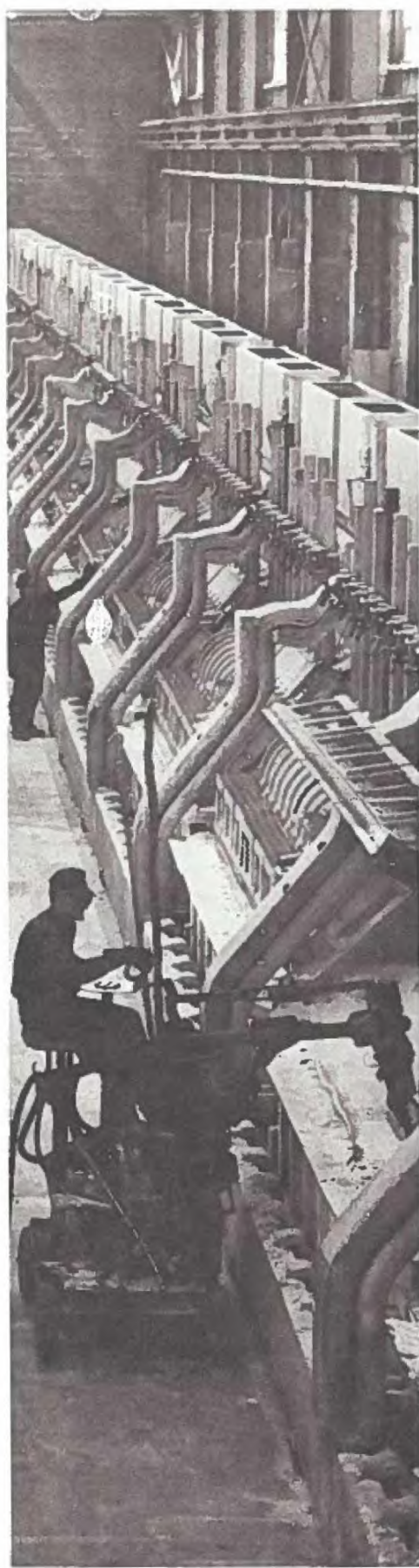
Worker uses a pneumatic crustbreaker to break the rock-hard crust which forms on the surface of the electrolyte bath at a modern aluminium smelting potline in Arvida, Quebec.
