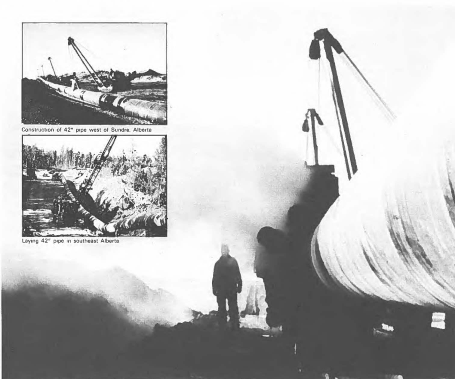
Coating and wrapping pipe for protection against corrosion PHOTOS: Alberta Gas Trunk Line Co.
