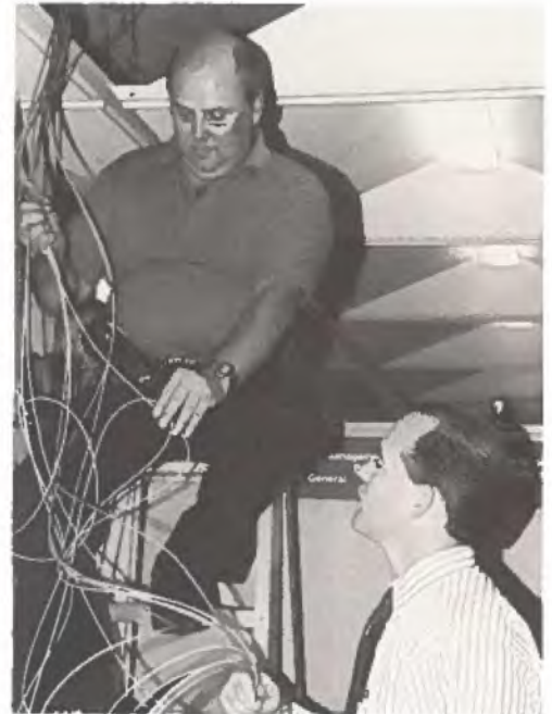
Cable inspection: Bert Bray (on ladder), DPW, and John Powell , Operations Officer, ASB.
