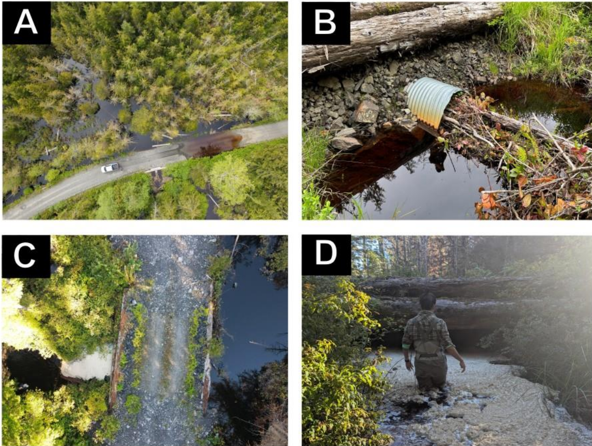
Figure 8. Photographs of flooding at road crossings in inlet (A and B) and outlet (C and D) streams of Misty Lake. (A) Aerial photo of flooding at inlet stream logging road crossing. (B) Obstructed culvert of inlet stream logging road crossing. (C) Aerial photo of flooding at outlet stream logging road crossing. (D) Collapsed log bridge of outlet logging road crossing. Photos taken by Paul Grant on May 22, 2025 (A), Scott Gilmore on May 22, 2025 (B) and September 17, 2025 (C), and Daniella LoScerbo on September 17, 2025 (D).
