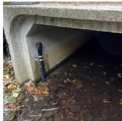
Figure 14: An ABS pipe housing a Solinst Levellogger 5 LTC logger, which is bolted to a culvert
