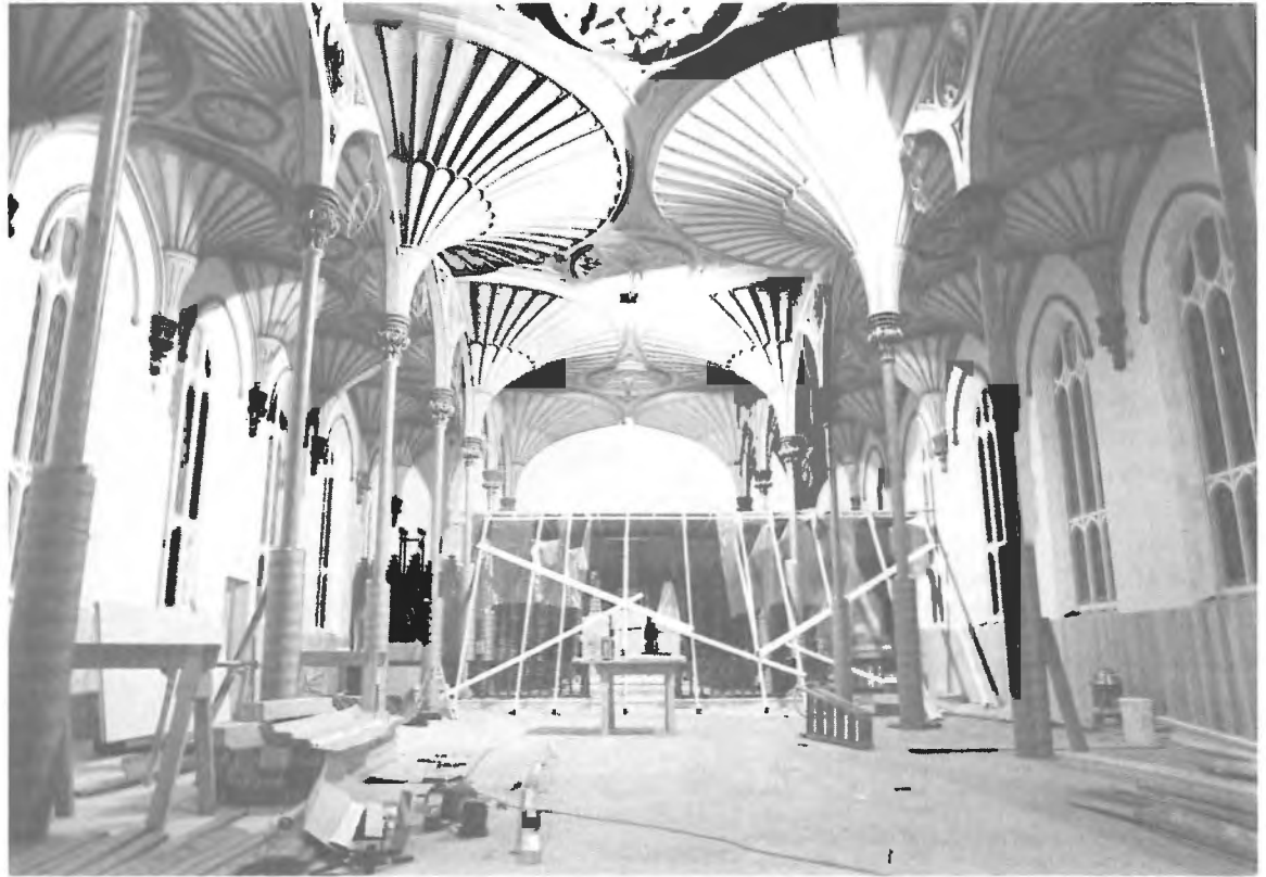
Installation of the timbers of the Rideau Chapel in the National Gallery of Canada.
