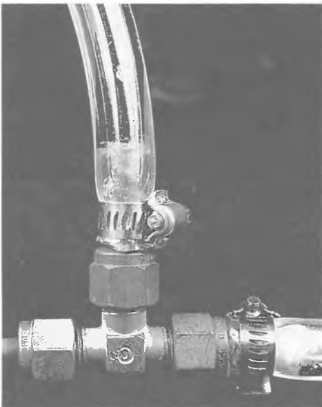
Figure 1. Green corrosion products produced where plasticized poly(vinyl chloride) tubing (Tygon) is attached to a brass fitting.
