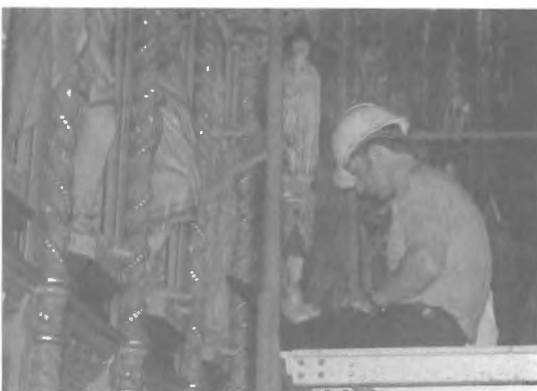
James Bourdeau carries out a condition survey of the interior of Notre-Dame Basilica in Ottawa.
