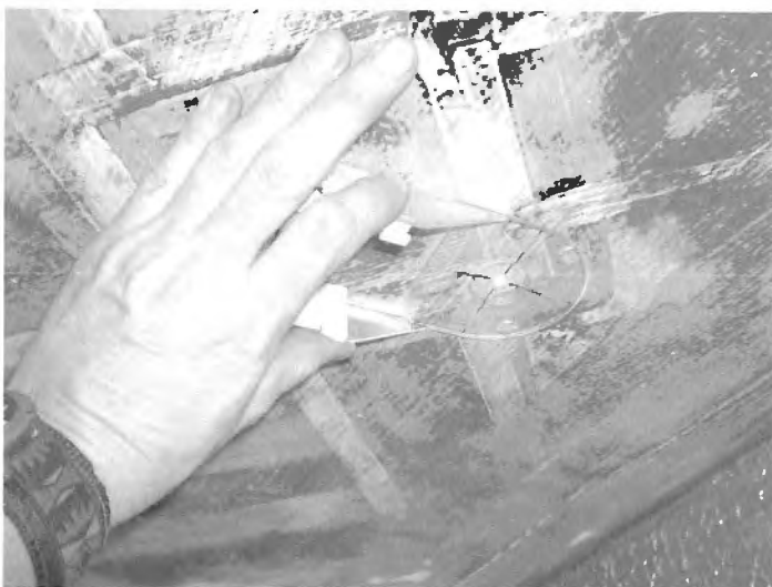
Original stencil pattern revealed below one of the 42 panelled areas on the ceiling of the Main Lobby. The target nozzle of the portable spectrophotometer is shown at a location where colour will be measured.
