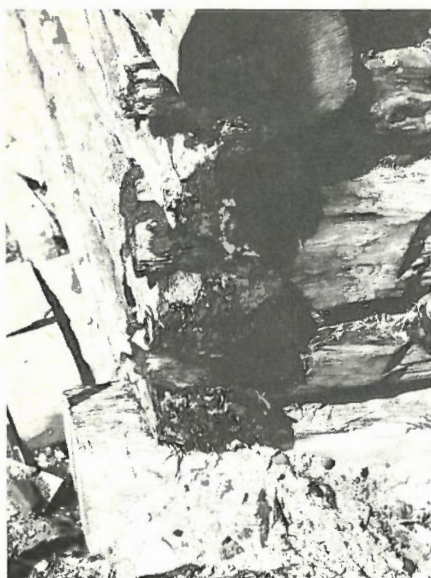
Example of typical wood decay in a log house. Acadian village of Caraquet, northern New Brunswick.
