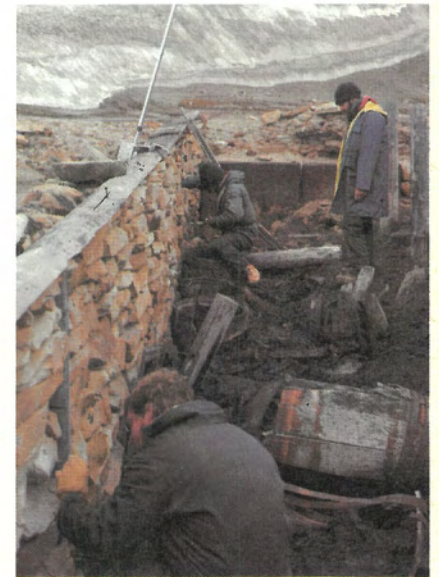
Bolt holes being drilled by hand in the sandstone drywall structure of Captain Kellett's cache on Dealey Island. The bolts will anchor the new floor to protect the artifacts which remain in situ.
