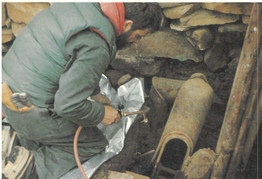
Occasionally a blow torch may be used to melt permafrost when excavating although hot water is more usual. In this work, ice around a cast iron ship's stove is being melted without direct heating of the stove itself.
