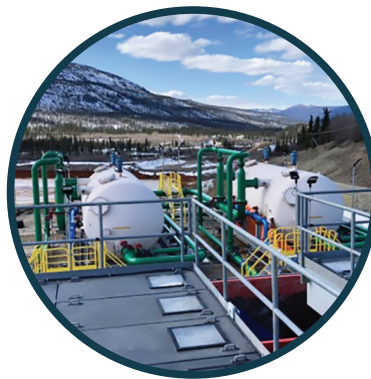
Cross Valley Pond Treatment Plant 10,902 m 3 /day
