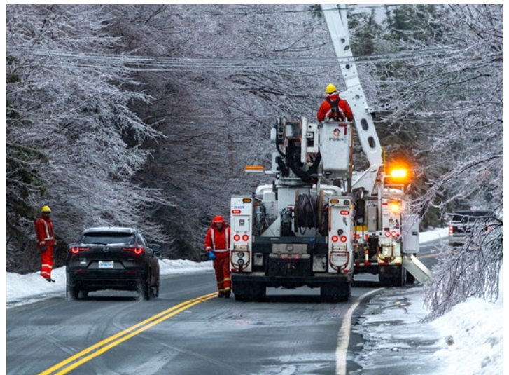
A power utility crew works to restore power after a damaging ice storm in Beaver Bank, Nova Scotia, on February 2, 2022.
