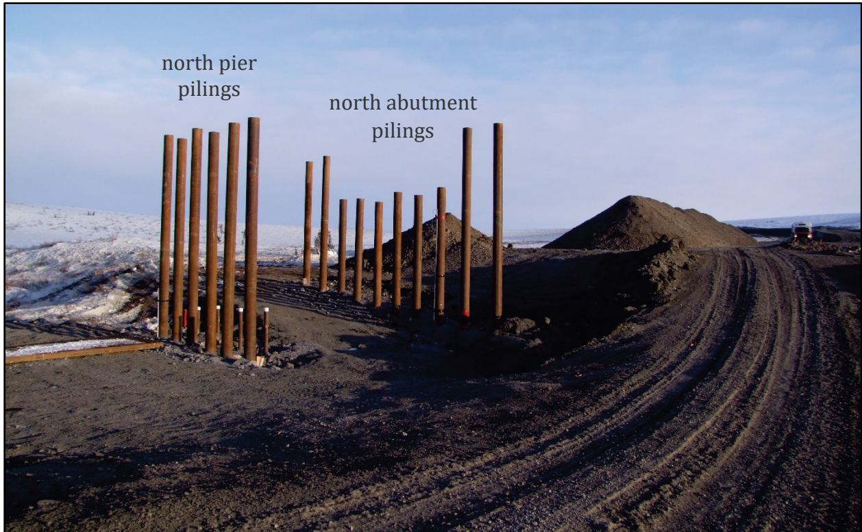
Figure 3. Northwest-facing view of the north half of the Bridge 23a site on 20 April 2016 during the NWT Permafrost Summit. The temporary road was built across the ice-covered stream.
