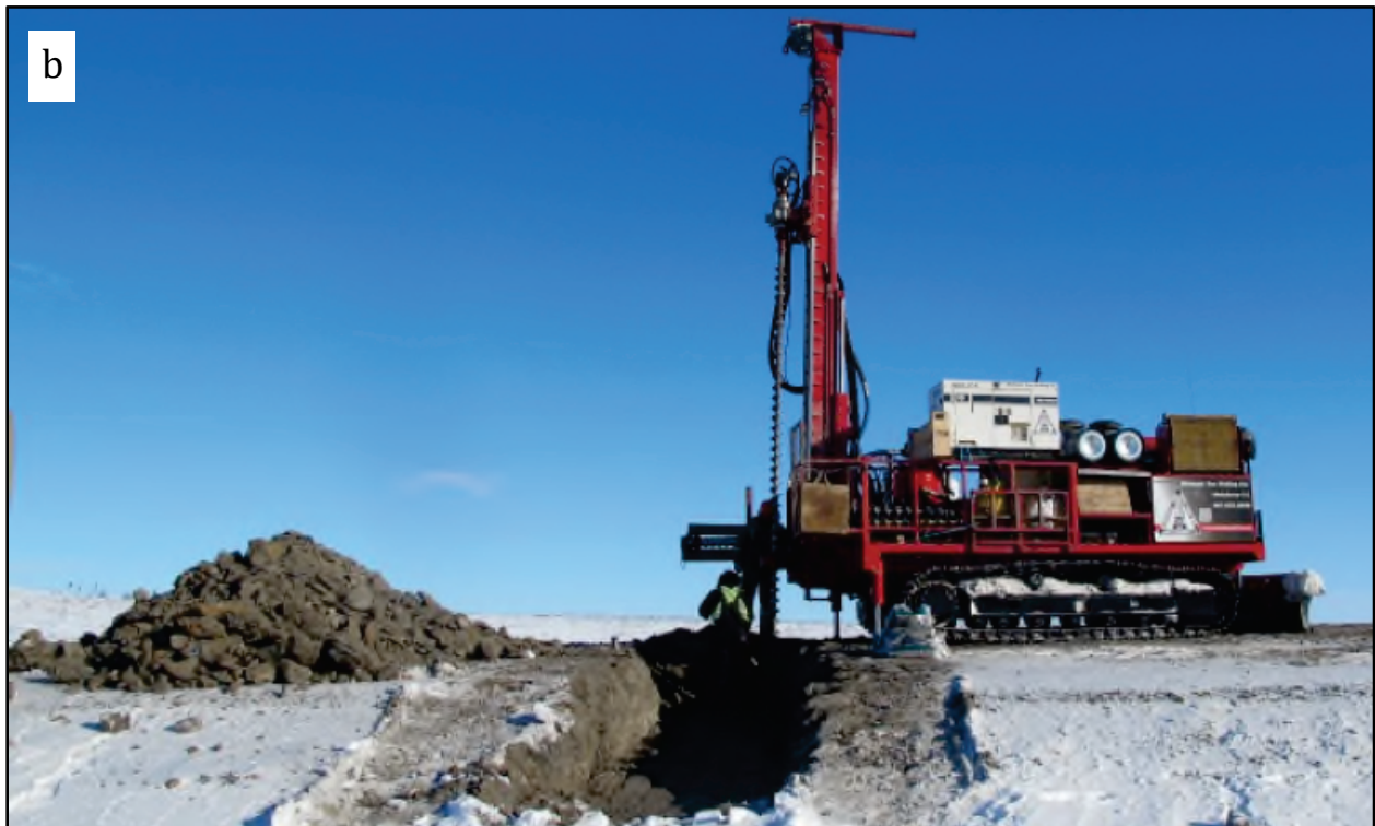
Figure 4. (a) Alignment borehole site AH18.15-S on 30 March 2013. Photo from Kiggiak-EBA (2013b). (b) Borehole drilling at ITH-4 following embankment excavation between foreground and embankment centre line. Photo from Kiggiak-EBA (2017b).
