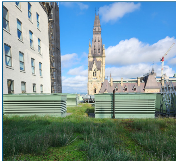
Figure 9: Configuration of mechanical systems during "as-operated" testing
