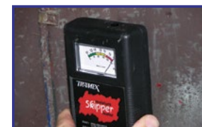
High moisture content
